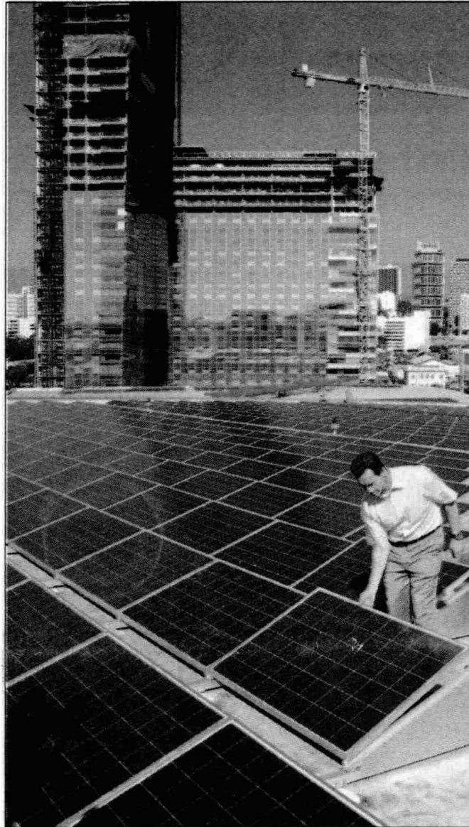
California Gov. Arnold Schwarzenegger examines the final solar panel modules on the roof of Staples Center's roof in Los Angeles on Tuesday, Oct. 28, 2008. The roof is now covered by approximately 24,196-square-feet of 1,727 solar panel modules.
